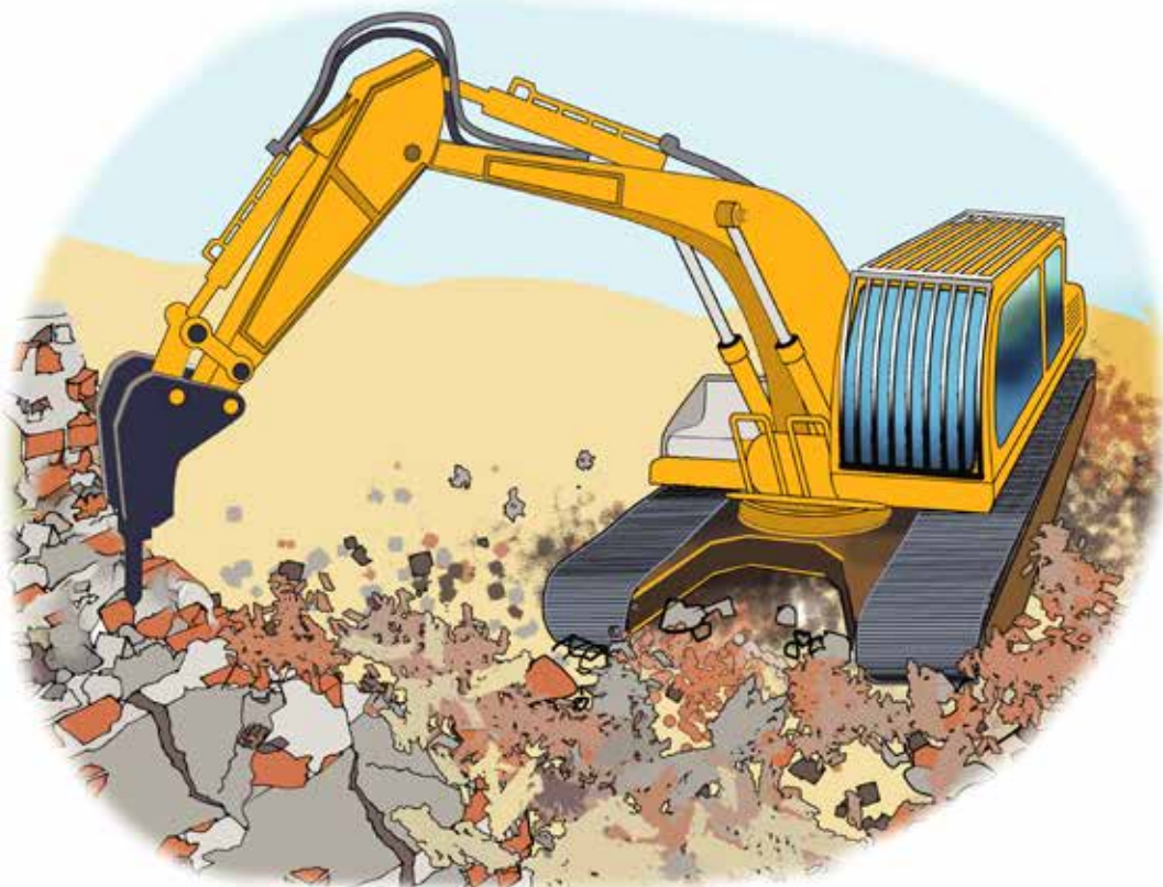
Figure 36.2. Mechanical demolition using an excavator is safer than manual demolition. Mechanical demolition requires adequate protection measures against falling objects.
