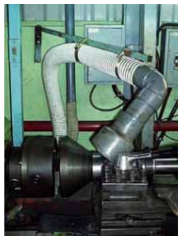
Simple local exhaust ventilation in a mechanical factory.
