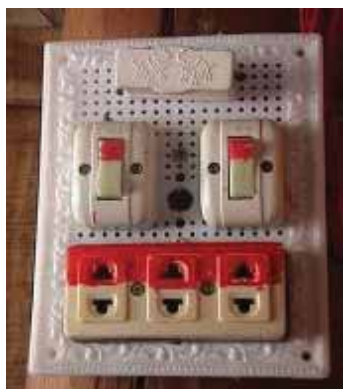
Use red color on the switches to make it clear what operation is intended.
