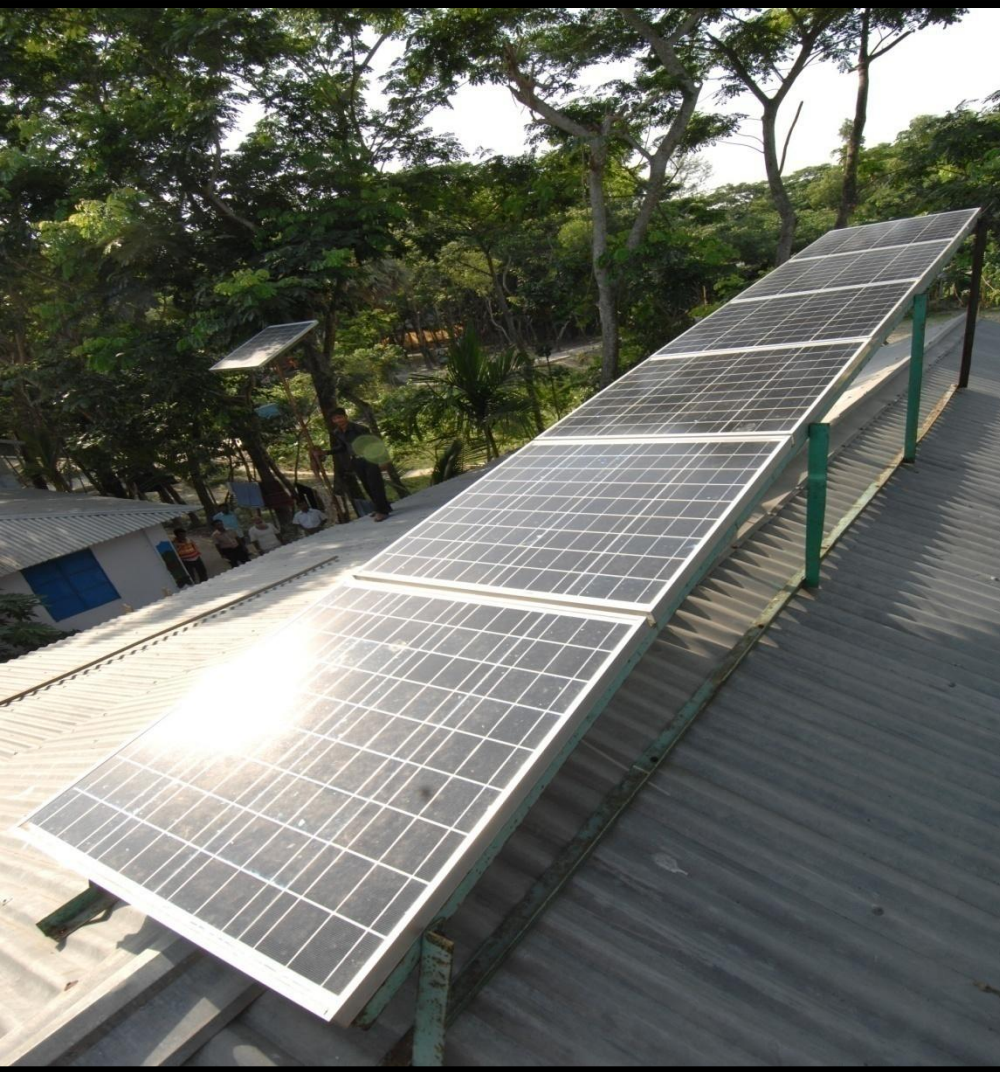
Solar panels on roof tops give power to computers
